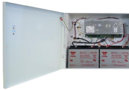
Figure 7 – Battery backup supply
