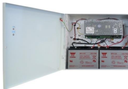
Figure 7 – Battery backup supply
