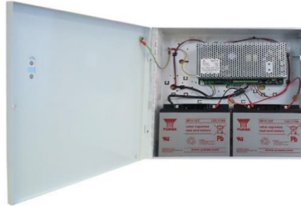
Figure 7 – Battery backup supply
