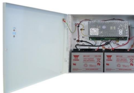
Figure 7 – Battery backup supply
